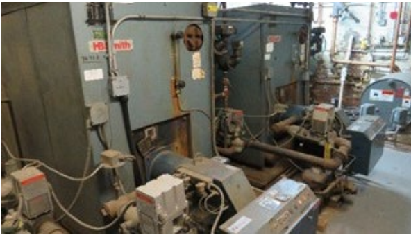
Hamilton Intermediate School - Boilers
