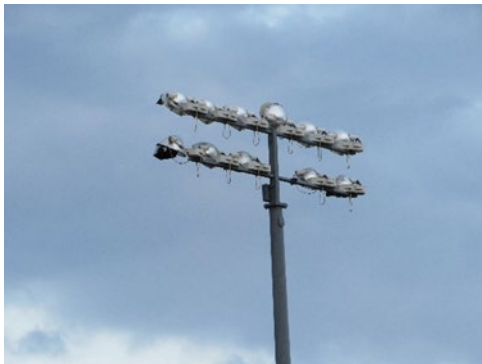
Harrison High School Stadium Field Lighting
