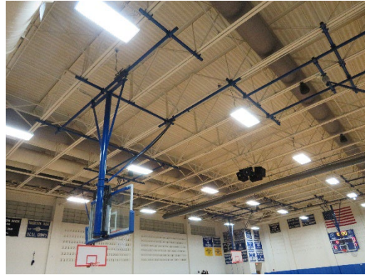
Existing Lighting at Harrison High School
