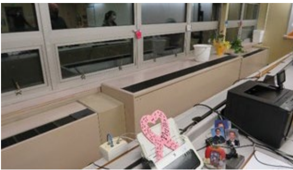
Washington MS – Typical Unit Ventilator
