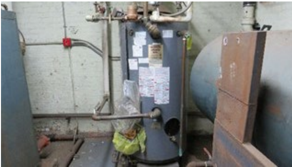
Hamilton Intermediate School Water Heater
