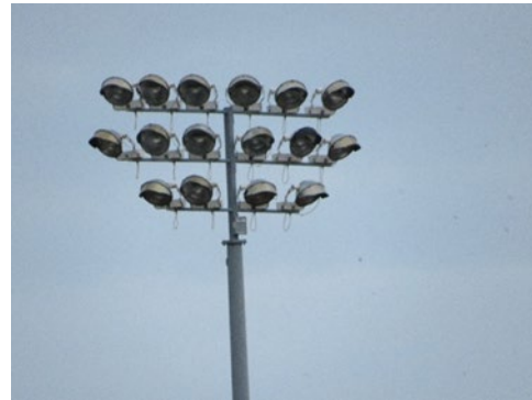
Harrison High School Stadium Field Lighting
