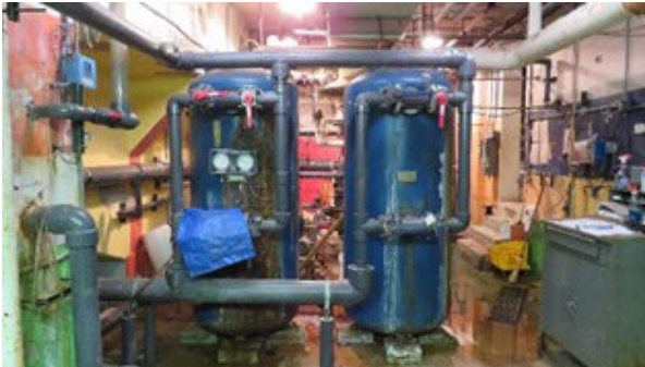
Washington MS Existing Pool Filters
