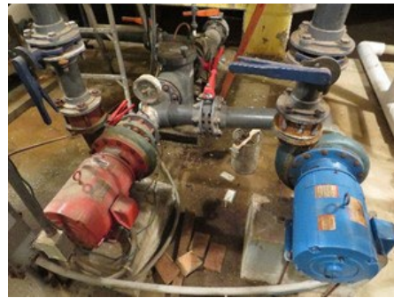
Washington MS Existing Pool Filter Pumps
