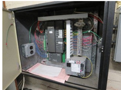
Lincoln School BMS Controller
