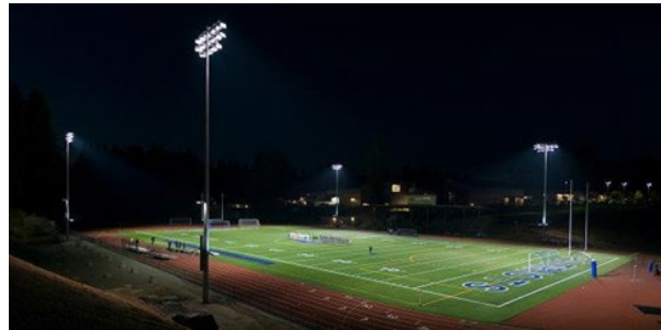
Example of Stadium Lighting
