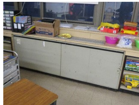
Lincoln ES – Typical Unit Ventilator
